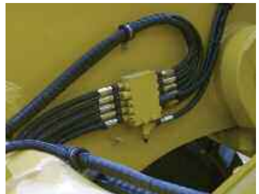
Lincoln system houses have experience to ensure installations are clean and neat
