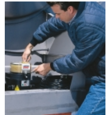
The QLS 301 is perfect for refrigeration and other types of trailers with a constant power supply.
