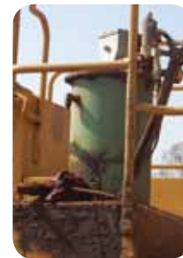
Over-filled reservoir with no overflow prevention system
