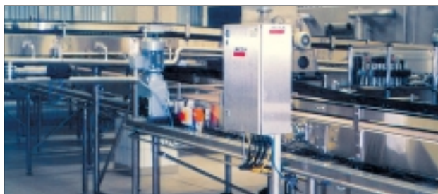
Section of a filling line with ejector cabinet
