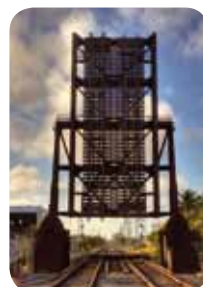
Auto lube systems on movable bridges
