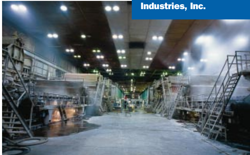
CHAMPION PERSONNEL INSTALLED SYSTEMS FOR MACHINES #3 AND #4 IN 1998.
