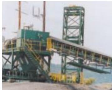
Belt transfer point uses a Quicklub® 203 electrical pump.
