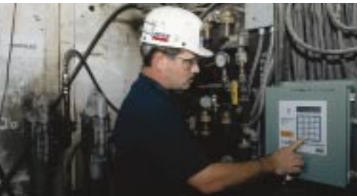
Kindill's giant Bucyrus dragline has four PowerMaster® pumps for more than 200 lube points. The lubricating process is controlled and monitored by a System Sentry unit. Jack Ellis, K&M Specialty Systems, checks the lube system before the machines move to a new position.
