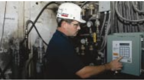
Kindill's giant Bucyrus dragline has four PowerMaster® pumps for more than 200 lube points. The lubricating process is controlled and monitored by a System Sentry unit. Jack Ellis, K&M Specialty Systems, checks the lube system before the machines move to a new position.
