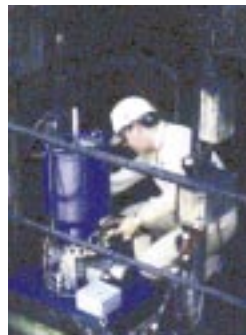
A competitor's lube system on a Ti-West rotary kiln faulted regularly; it was replaced by a Lincoln Industrial Multi-Line 215 pump controlled by a System Sentry II.
