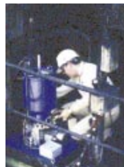
A competitor's lube system on a Ti-West rotary kiln faulted regularly; it was replaced by a Lincoln Industrial Multi-Line 215 pump controlled by a System Sentry II.
